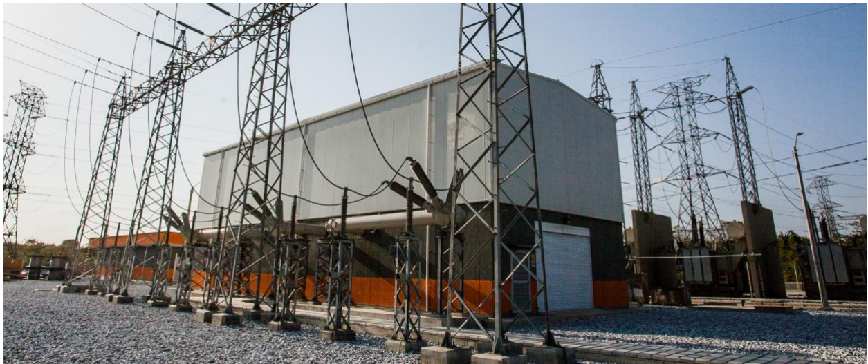
▶ Caracolí Celisa Substation Atlántico, Colombia
