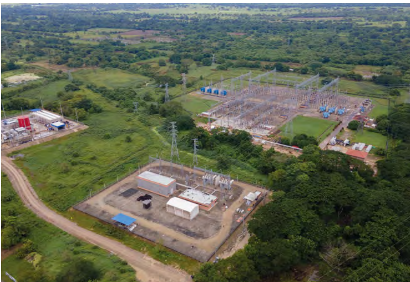
Bolívar Substation Bolívar
