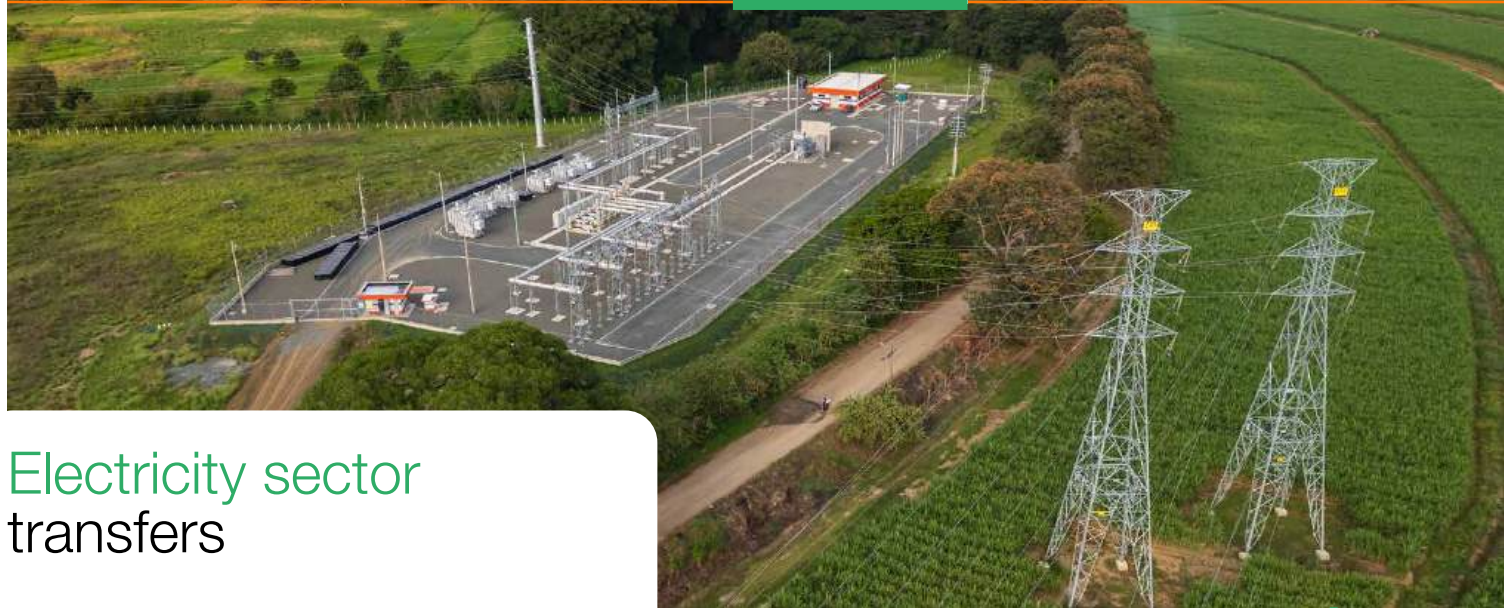
Istanbul Substation, Valle del Cauca.
