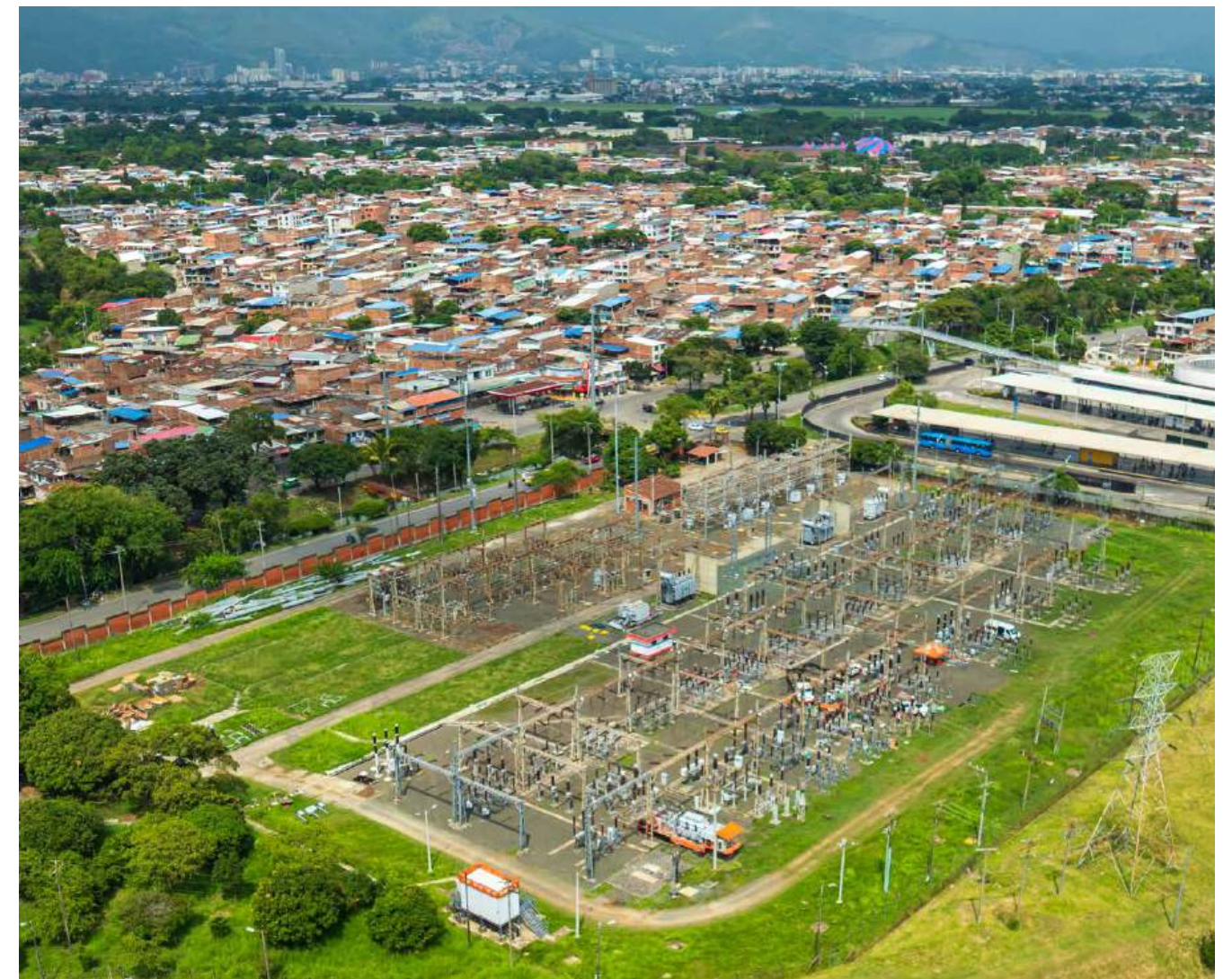
Juanchito 115 kV Substation, Cali, Valle del Cauca.
