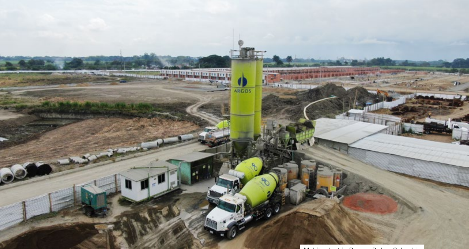
Mobile plant in Parque Dulce, Colombia
