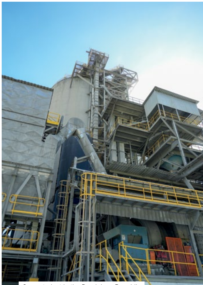
Cement plant in the Dominican Republic
